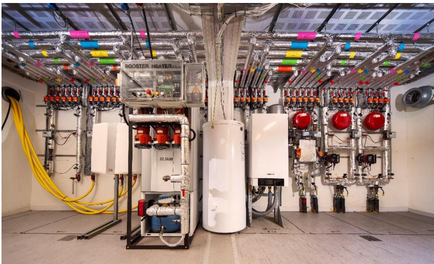
Picture 4. Flexible District Heat integration at SYSLAB Facilities
