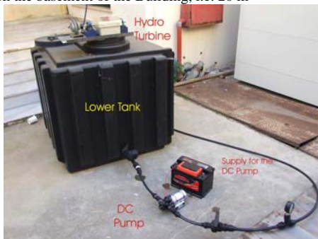
The lower Tank and the infrastructures for pump storage
